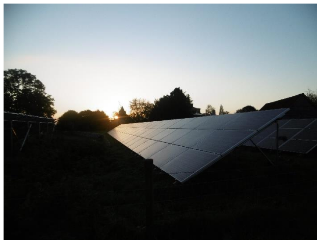
Figure 6-6: Solar PV array at Canon Frome Court cohousing
