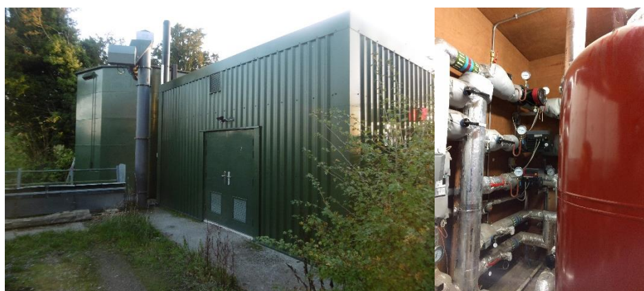
Figure 6-4: Canon Frome Court cohousing's biomass boiler, exterior and interior
