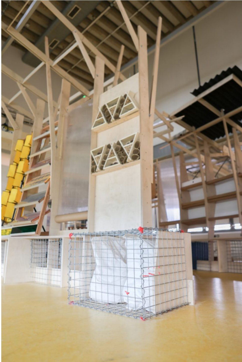
Architects for Gaza has created a 1:1 prototype of a healthcare clinic for Gaza
