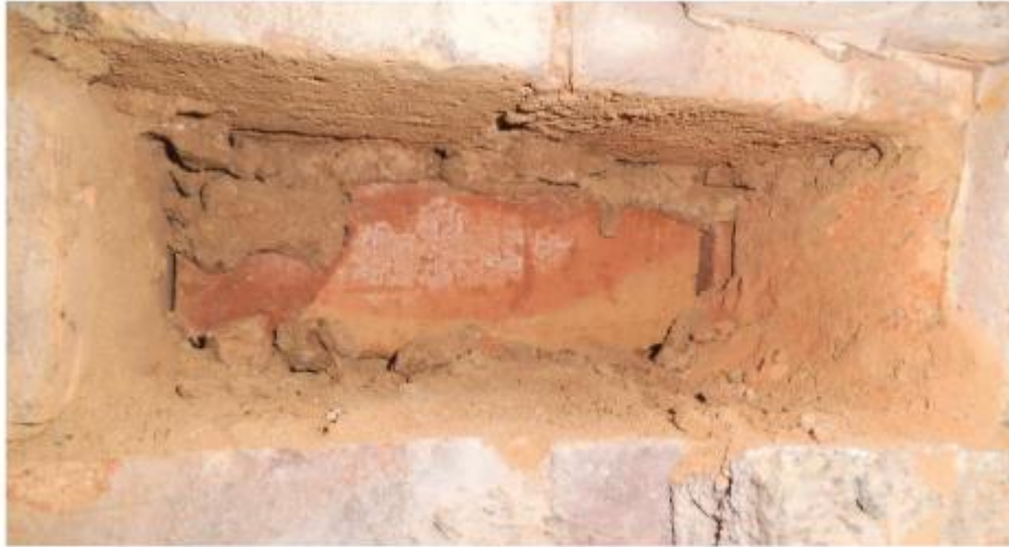
Figure 1: An example of the space revealed inside a solid wall following the removal of a 'stretcher' brick, from Report 2. The joint between the two stretcher bricks (known as the 'collar joint') shows little evidence of mortar; the lack of staining across most of its surface indicates that no mortar was present in this space. This air space is likely to significantly increase the thermal resistance, and reduce the Wall U-value.
