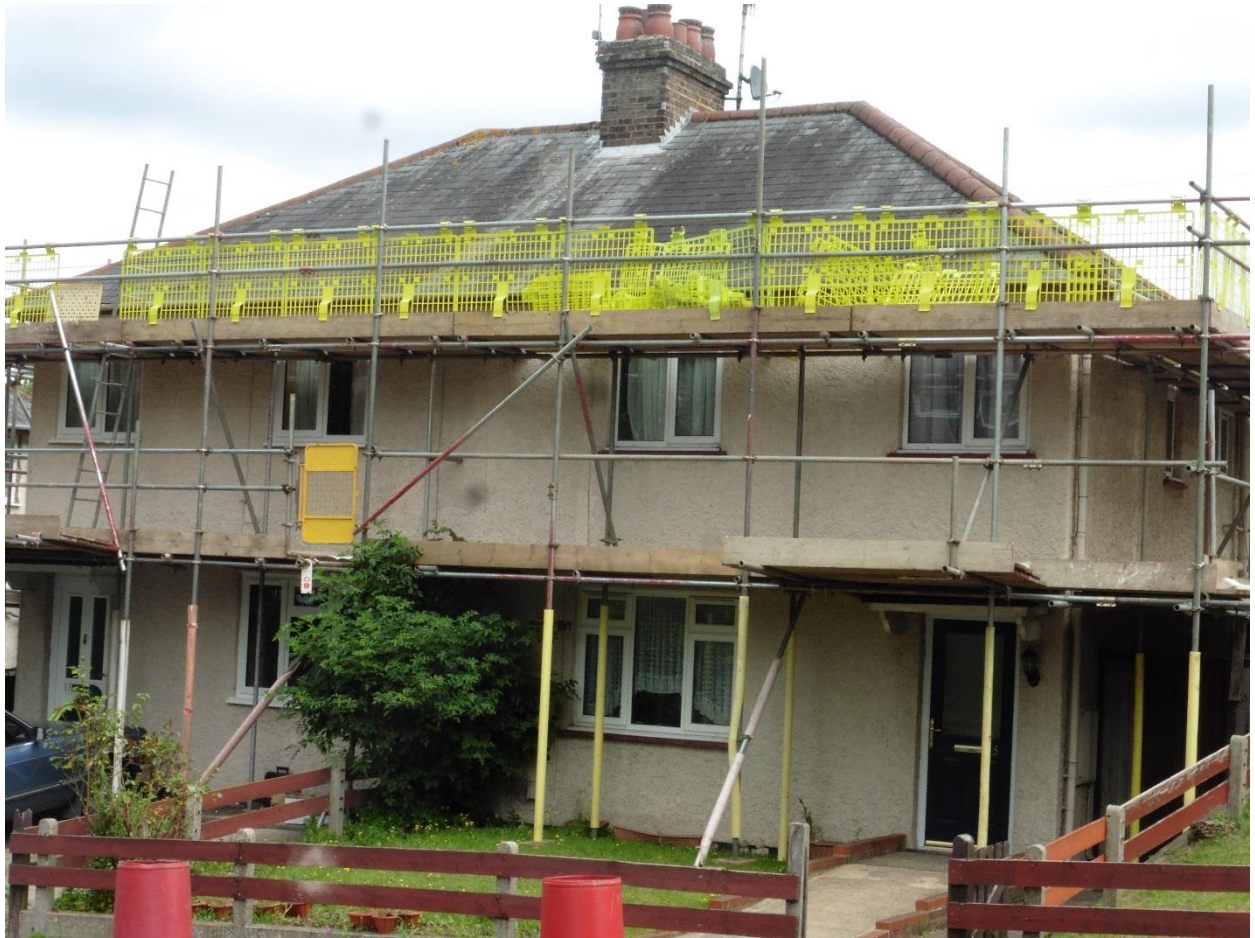
Figure 62: Dwellings 2 and 3 visited for moisture dust drillings.
