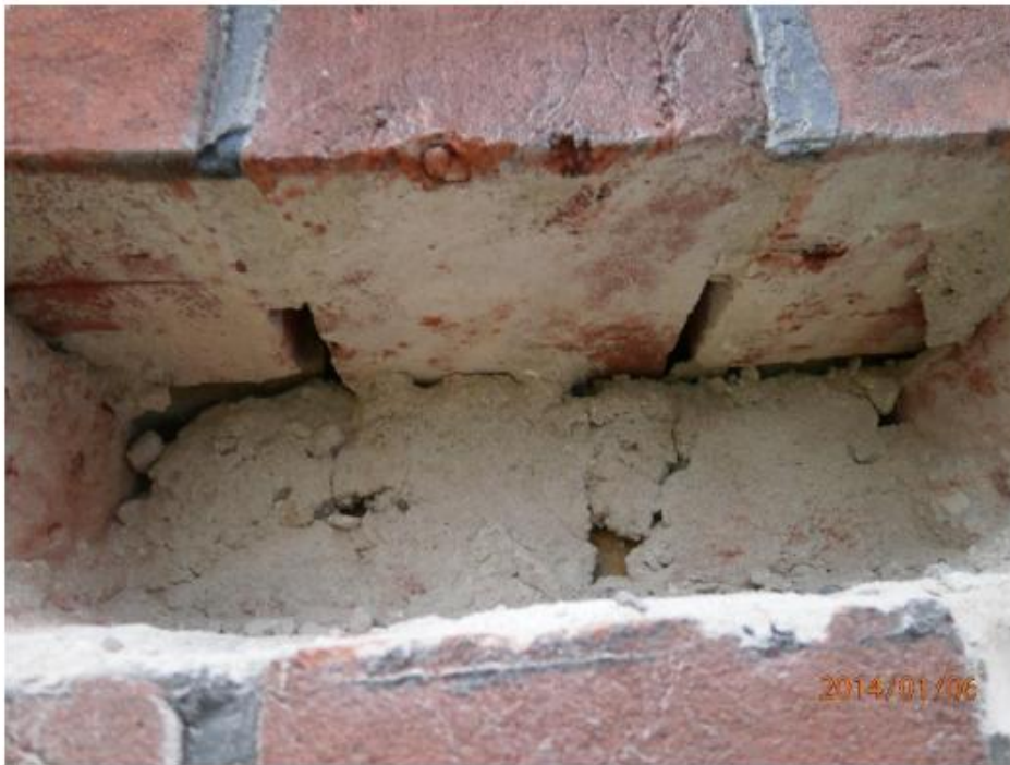
Figure 8: Example of missing mortar in perpend joints. Looking upwards at exposed bricks in the upper course at the top of the void, the extent of mortar in the perpend joints can be seen. In this example, the perpends can be estimated to be approximately 50% filled.
