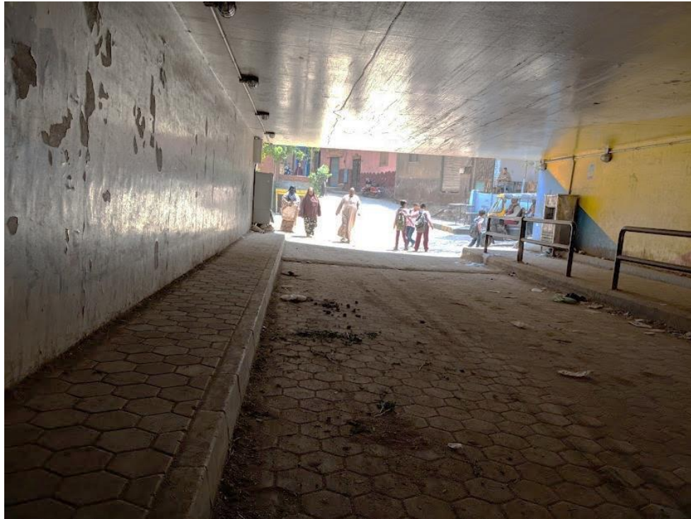
Figure 7.17 The underpass and the mural showing signs of degradation two years after the intervention (source: author)
