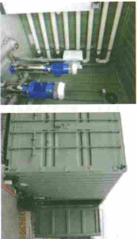
Figure 2: A mobile water treatment system is one possible temporary infrastructure use for shipping containers
