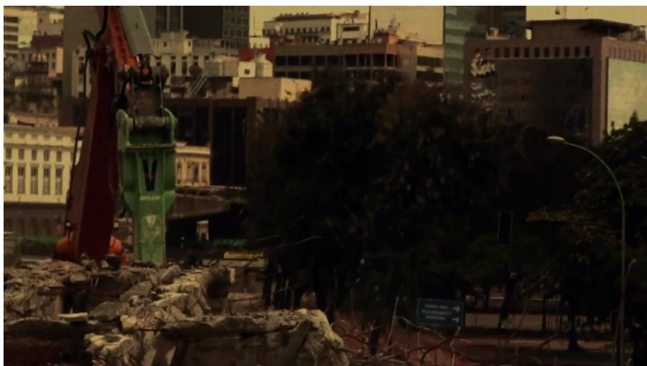
Figures 38, 39, 40 and 41 – The debris of the Elevado da Perimetral in ExPerimetral
